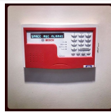
SMOKE AND FIRE ALARM : OFFICE SPACE
