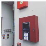
SMOKE AND FIRE ALARM : RESTAURANT
