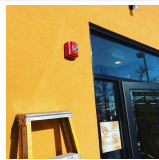
SMOKE AND FIRE ALARM : RESTAURANT
